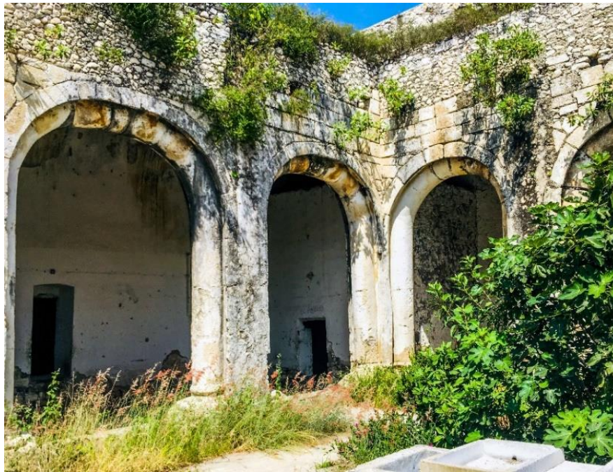
Figure 14: The cloister of the la Comunidad complex. Photograph in the collection of Robert H. Jackson.
