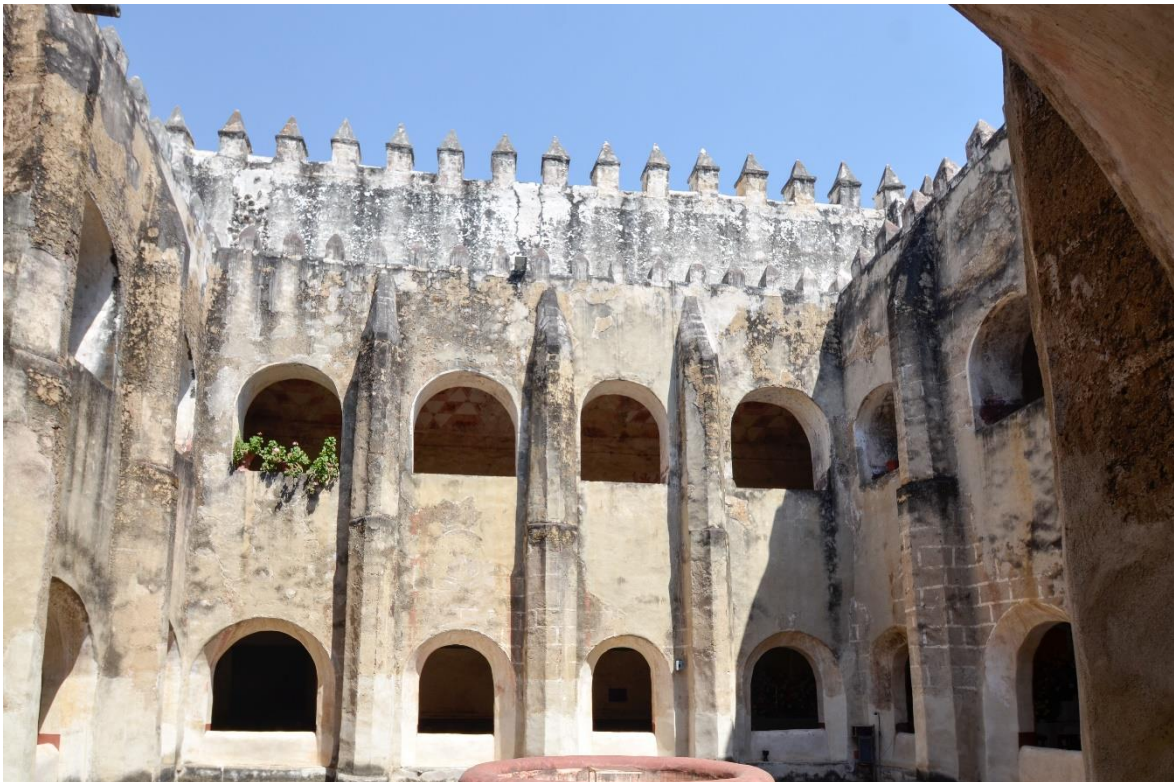
Figure 28: The cloister of the doctrina complex. Photograph in the collection of Robert H. Jackson.
